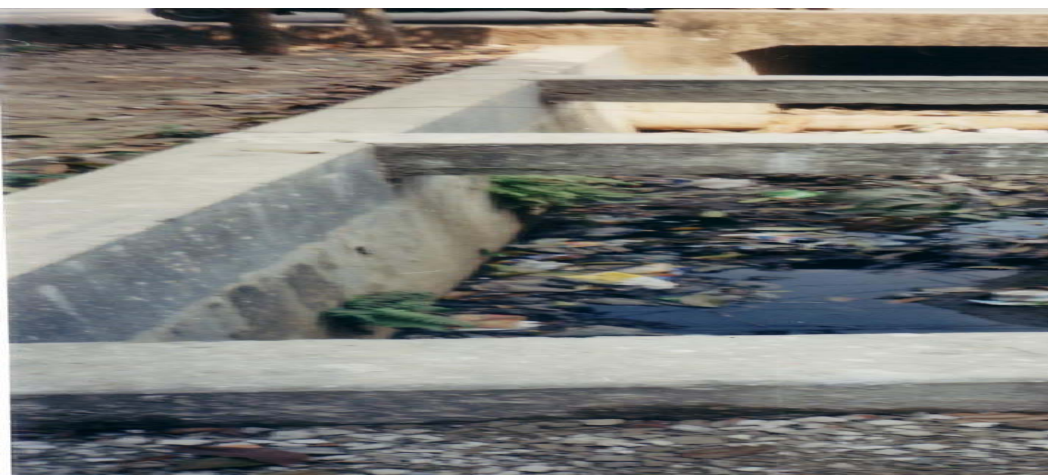
Figure-4. Drain blocked by solid waste at Pathantula.
