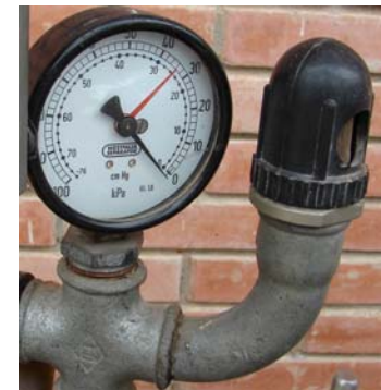
Vacuum gauge and control valve
