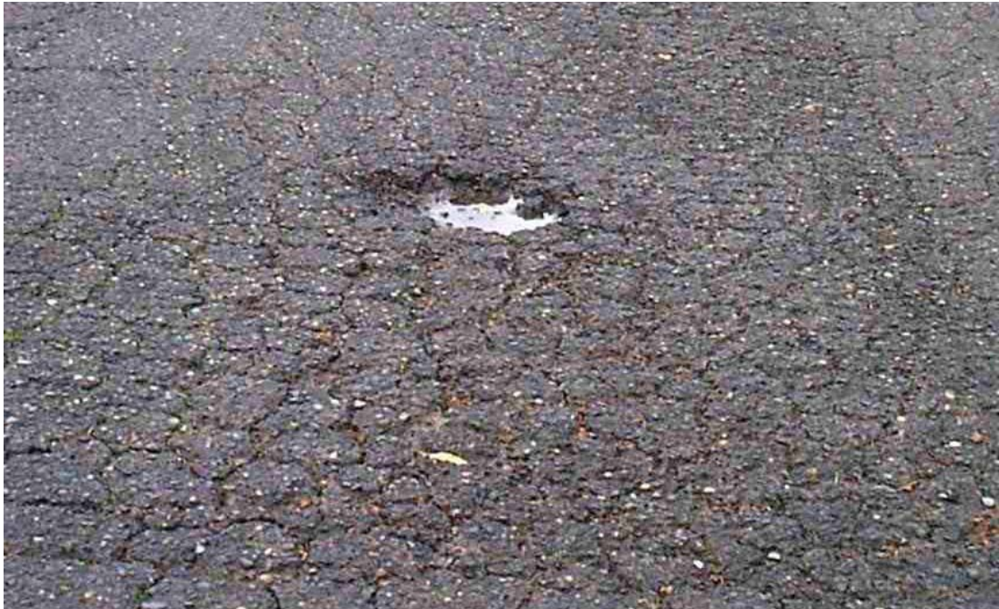
Figure-3. Pothole distress repair by replaces some or the entire granular layer.
