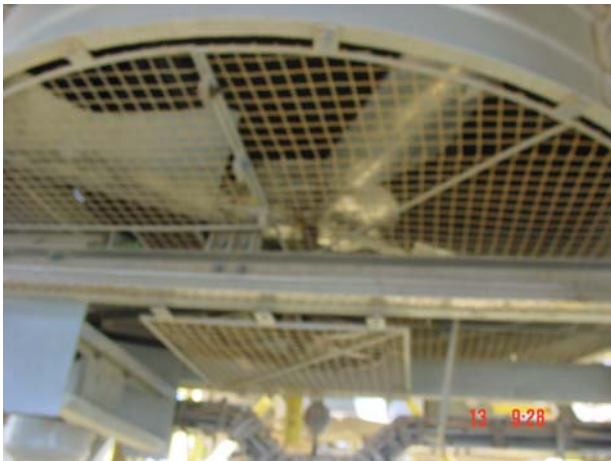
Figure-2. General view of plenum with blades inside.
