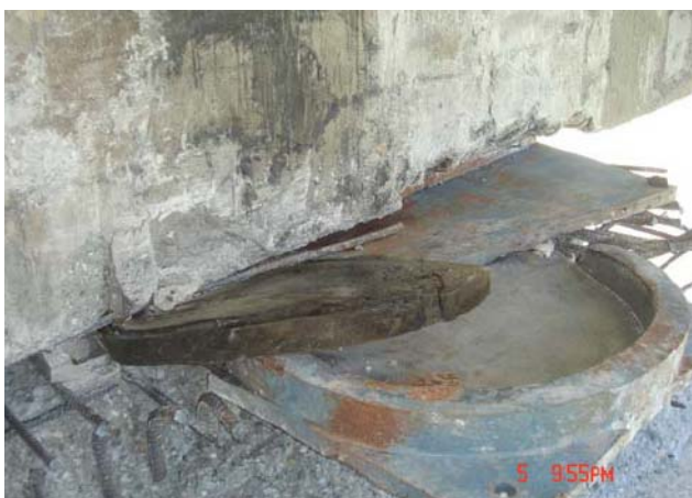
Figure-5. Damage of support.
