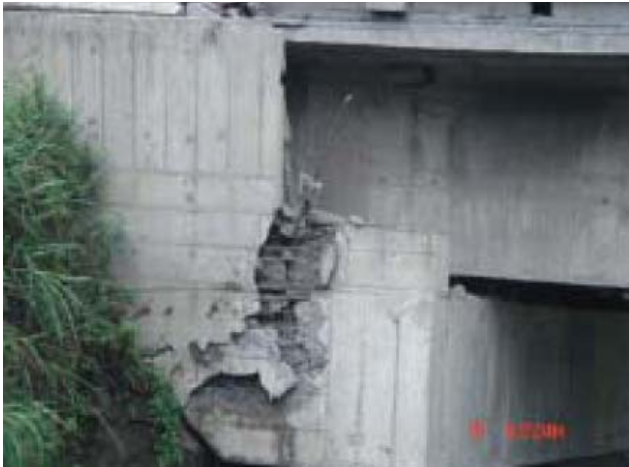
Figure-3. Damage of abutment.
