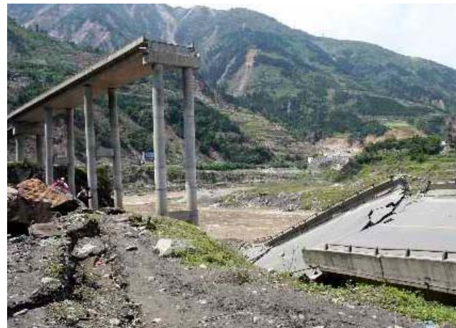
Figure-6. Damage of main beam.
