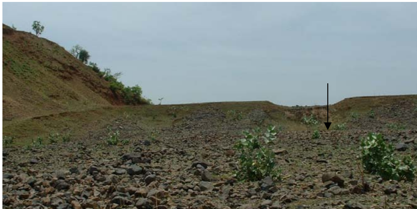
Plate-4. Land slide (Slope failure) near the right abutment.
