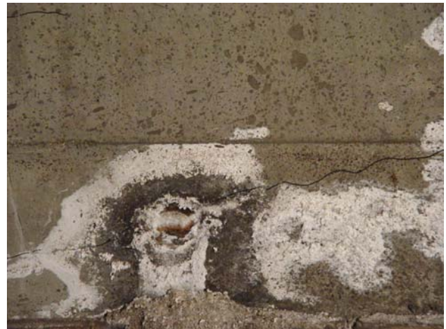
Figure-7. Damage of seepage in concrete.
