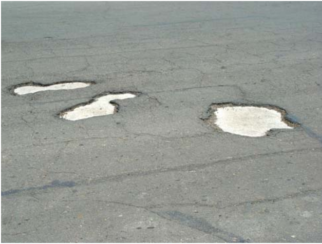
Figure-3. Damage of deck pavement.
