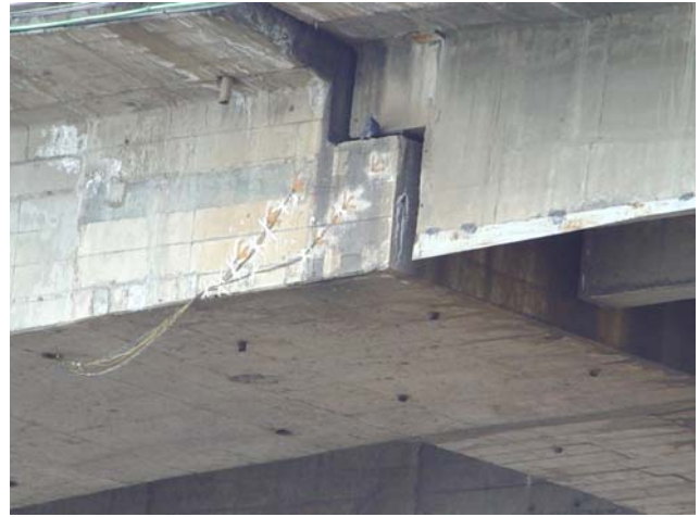
Figure-6. Damage of corbel
