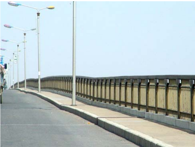
Figure-4. Down deflection of the bridge.
