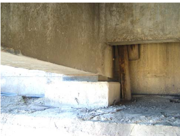
Figure-5. Damage of bearings.
