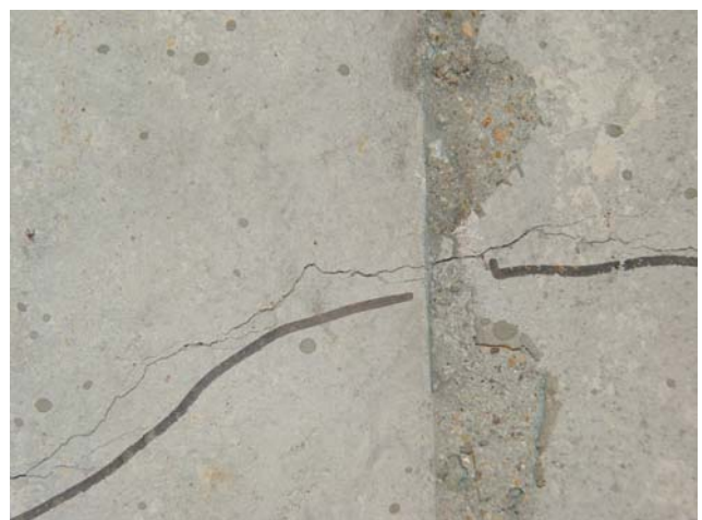
Figure-8. Cracks in concrete.
