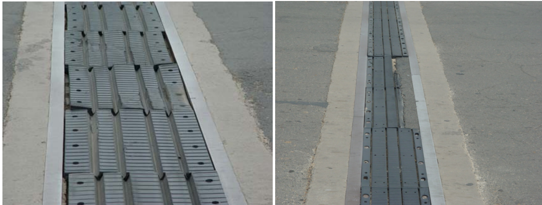
Figure-9. Damage of expansion joint.
