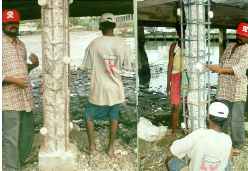
Figure-11. Typical position of galvanic anode and application of zinc rich primer.
