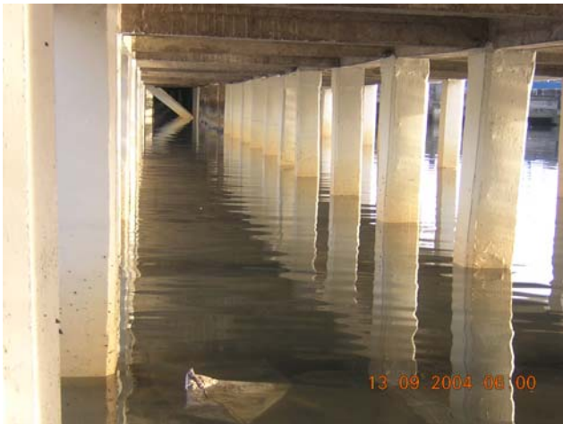
Figure-13. A complete view after the jacketing with under water micro concrete.
