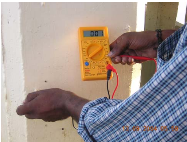
Figure-14. A view of the half cell potential test after the rehabilitation.
