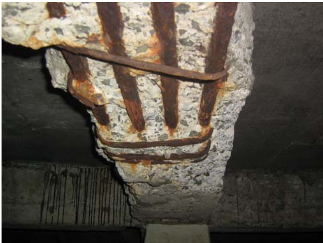
Figure-9. Typical view of the corroded/spalled beam.
