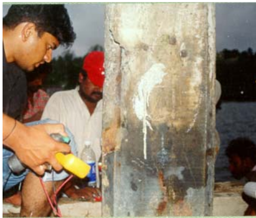
Figure-10. A view of the half cell potential test in progress on the pile before rehabilitation.
