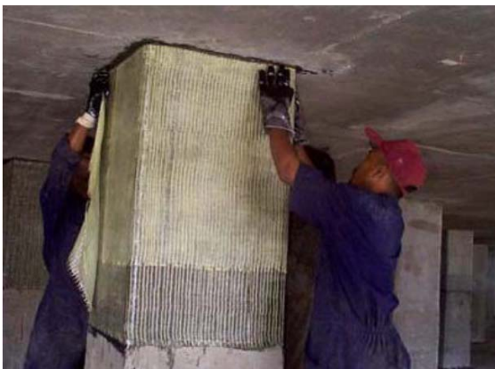
Figure-2. Seismic retrofit of supporting columns for a cryogenic tank in Gujarat, India
