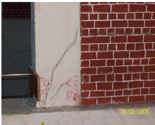
Figure-11. Crack in leeward column.
