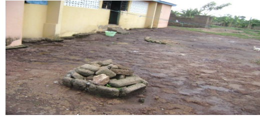
Figure-9. Eroded topsoil in the sumampa catchment.
