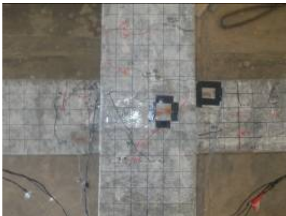
Figure-11. Crack pattern of MC specimen.
