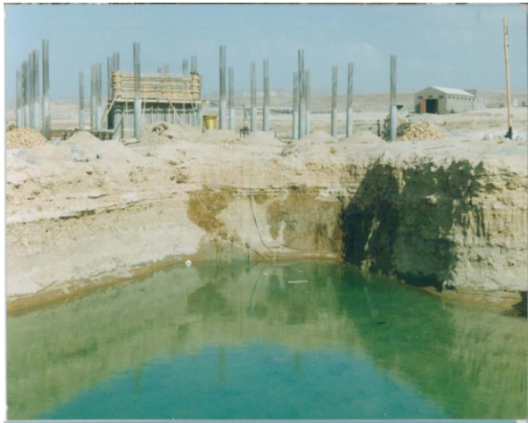
Figure-2. Lack of geo-technique experiments and construction in unsuitable place.
