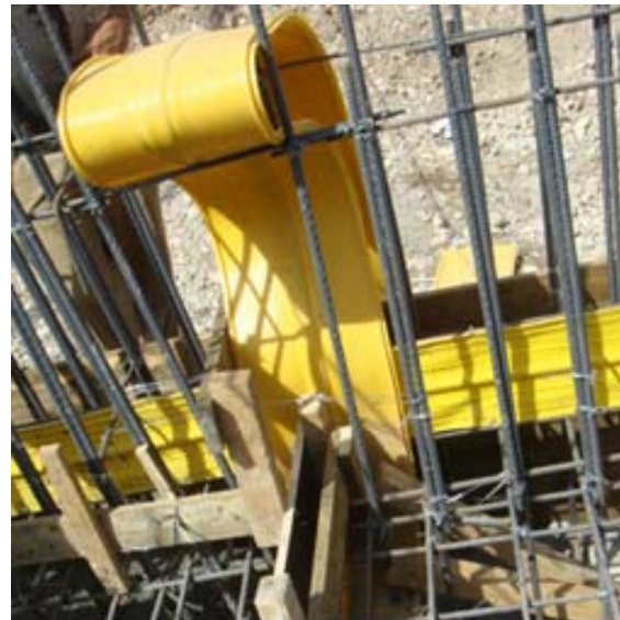
Figure-13. Rubber of expansion joints used for construction joints in the Bawashaswar bottom outlet gallery.
