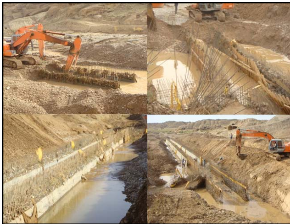
Figure-12. Effect of flood on bottom outlet gallery of Bawashaswar dam.
