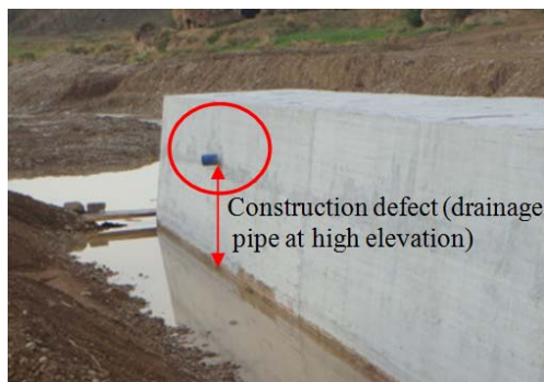
Figure-5. Location of the drainage pipes at Bawashaswar dam.
