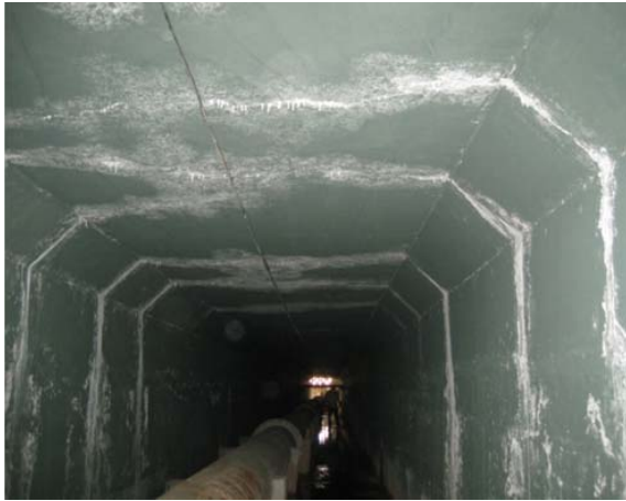
Figure-14. Residues of seepage at fractures along the bottom outlet gallery.
