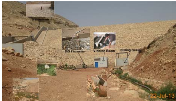
Figure-8. Seepage at Hamamuk dam site.
