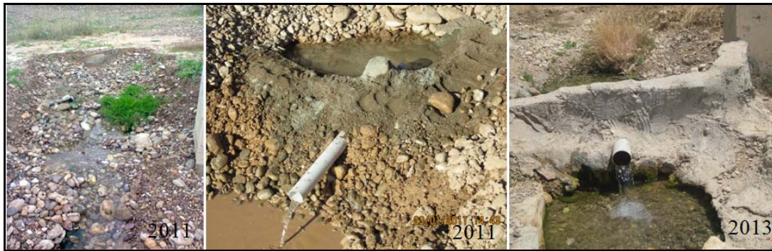
Figure-4. Seepage at the downstream flat slope of Bawashaswar dam.
