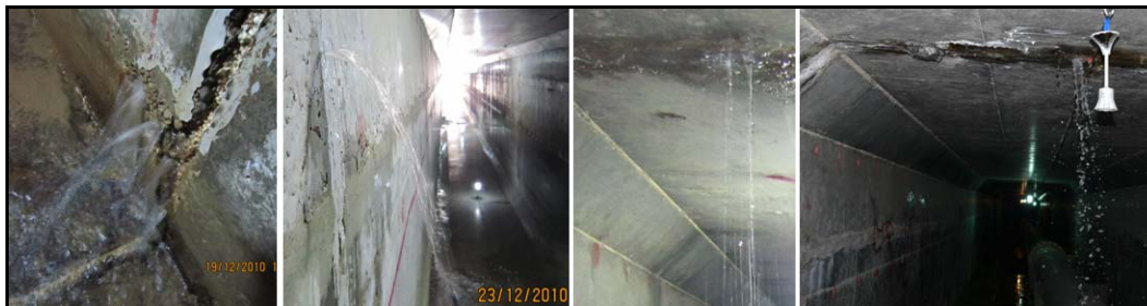
Figure-3. Seepage at the expansion and construction joints of the outlet gallery of Bawashaswar dam.
