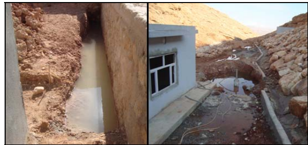
Figure-16. Seepage at Hamamuk dam during initial filling.
