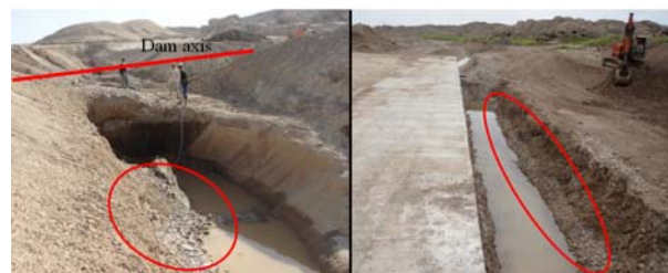
Figure-9. Recent deposits at downstream shell foundation of Bawashaswar dam.
