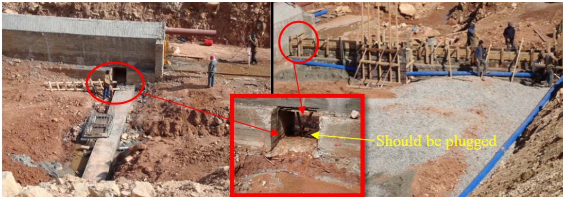
Figure-17. Defect at drainage system of Hamamuk dam.
