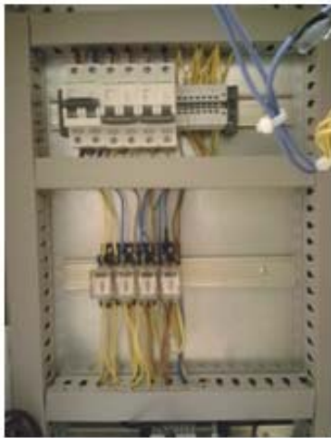
Figure-6. Control Box Wiring.
